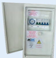
SBX-5 cover removed
